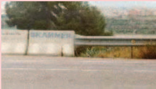
Wrong joining between barriers
